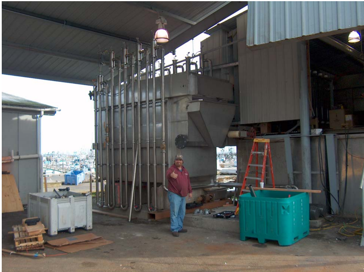
Figure 9. Actual photo of the wastewater treatment system at the Ocean Gold plant.
